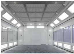
Painting booth/ Air make up system
