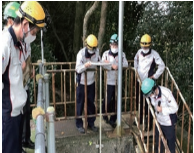
Training for opening and closing of valve in front of discharge port
